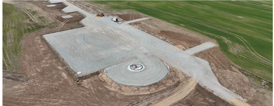
The picture shows hardened surfaces and concrete foundations of the Pienava wind power project (147 MW) in the municipality of Tukums, Latvia. The project entered the construction phase in connection with the sale to Latvenergo in July 2025 and is expected to be completed in 2027.
